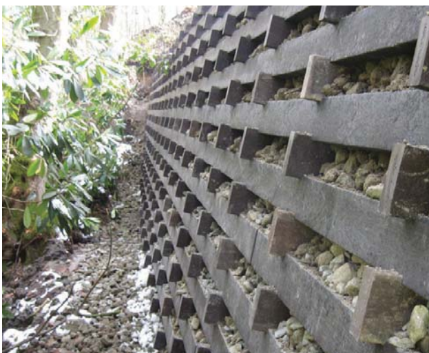
The EcoCrib™ facing offers an aesthetically pleasing and durable facing that blends into the natural surroundings.
