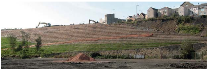
Construction using standard equipment and materials keeps cost and time to a minimum.
