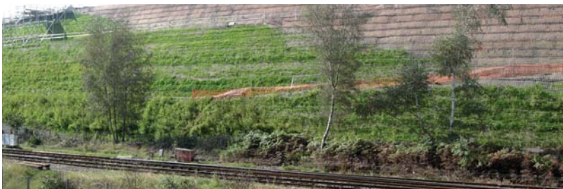
With construction successfully completed, the TensarTech GreenSlope is ready for the vegetation stage.
